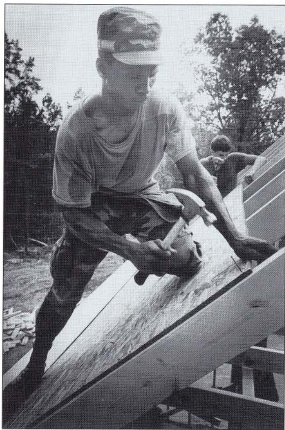
Fig. 10. The Mississippi National Guard selected the Field Station as one of their public service projects in 1990 and 1991. One of the guardsmen is constructing the roof on the station manager's home.
